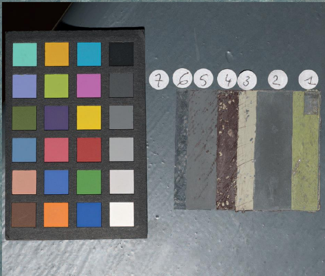
Areas of uncovering showing successive paint layers applied after the construction of the show flat in La Cité Radieuse by Le Corbusier, Marseille (France), 1952; Photo: 2015, CICRP(Odile Guillon); Weyer, E. (ed.), (2015), EwaGlos:European Illustrated Glossary Of Conservation Terms For Wall Paintings And Architectural Surfaces, Petersberg: Hornemann Institute; 248.
