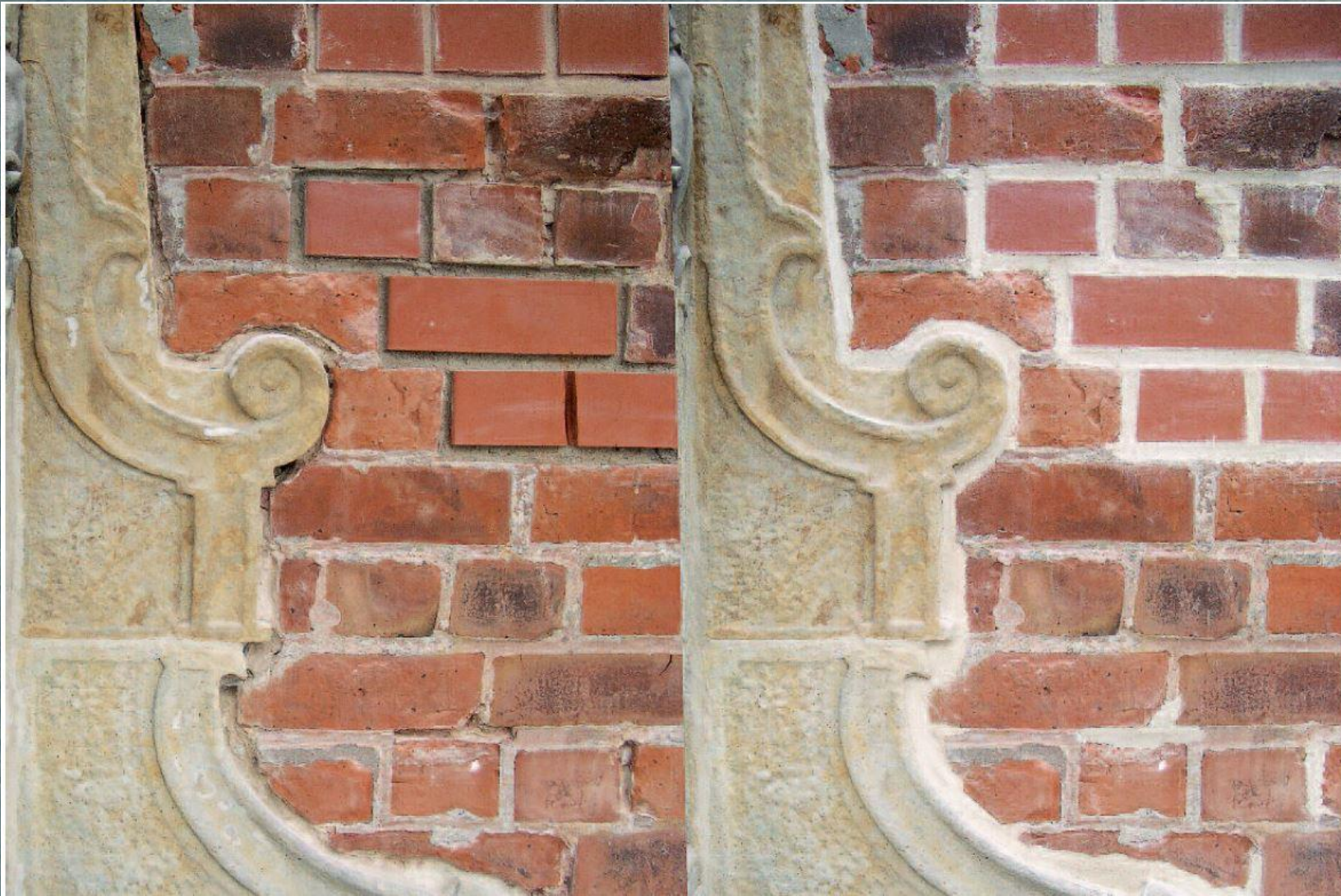
Raked (left) and repointed joints (right) of brick masonry and parts of a sandstone epitaph, Church of St. Gabriel, Haseldorf (Germany), end of 16th century; Photo: 2007 (Sophie Haake); Weyer, E. (ed.), (2015), EwaGlos:European Illustrated Glossary Of Conservation Terms For Wall Paintings And Architectural Surfaces, Petersberg: Hornemann Institute; 320.
