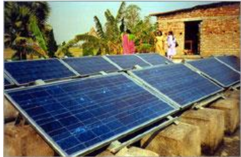
Rooftop PV modules on a village
