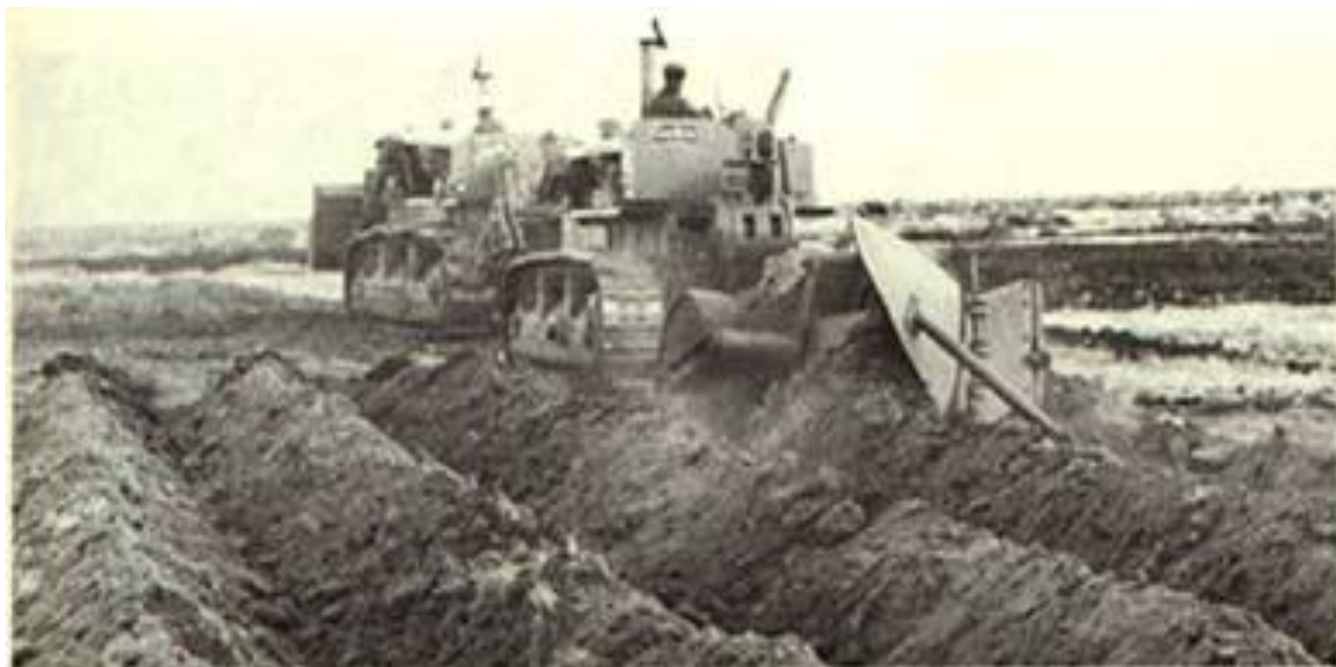
Figure 5. Moldboard plowing three feet deep in stratified soil. Pre-ripping is sometimes necessary in hard soil.
