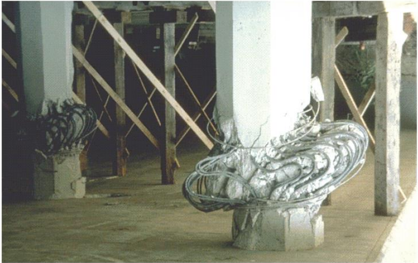
Column failure on interstate highway overpass, Northridge earthquake. (Photo from: http://earthquake.usgs.gov/bytopic/photos.html )
