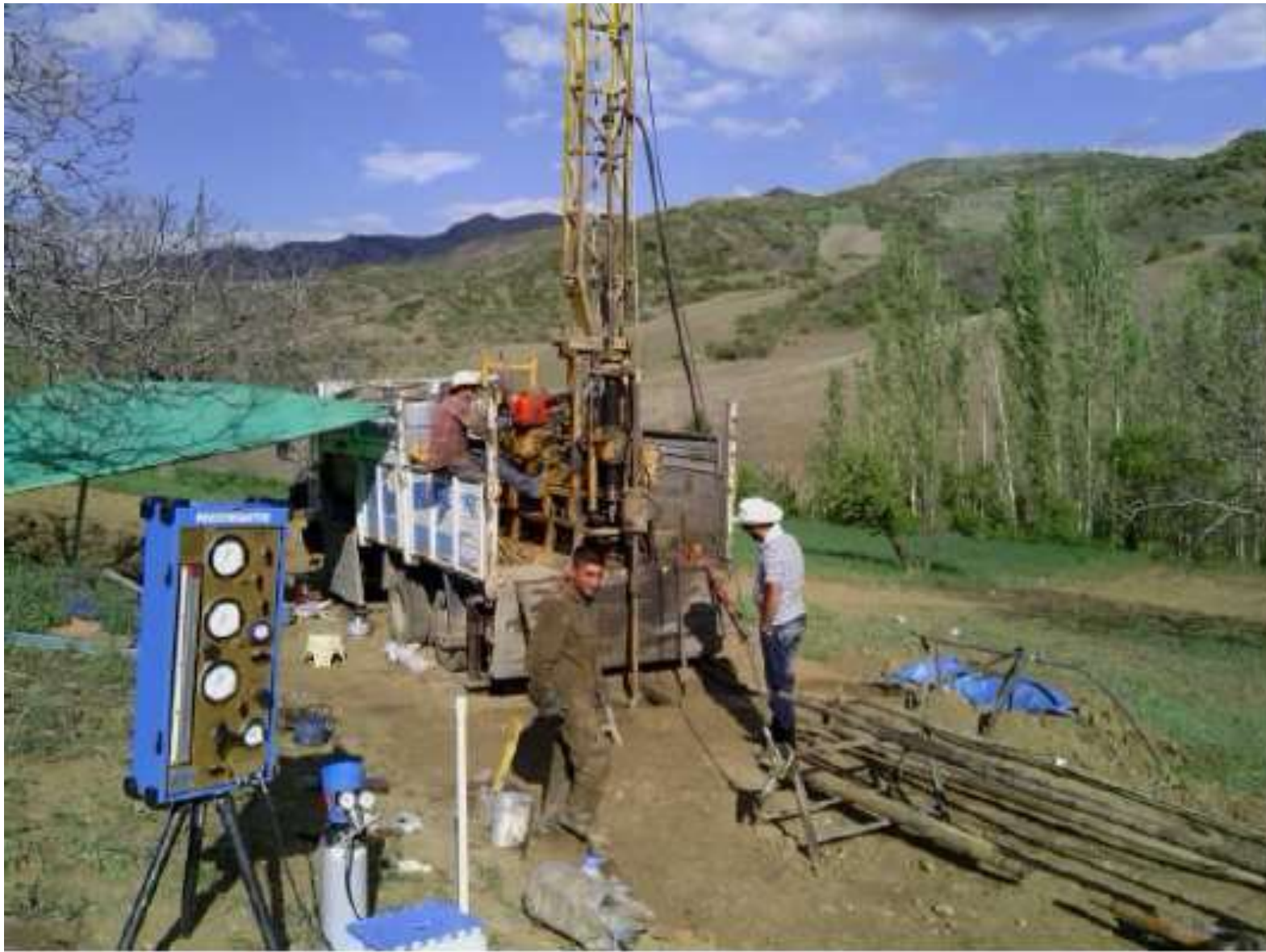
Field instrumentation of soil material at Çorum-İskilip Reservoir/dam site (Photo courtesy of Alter, 2014)
