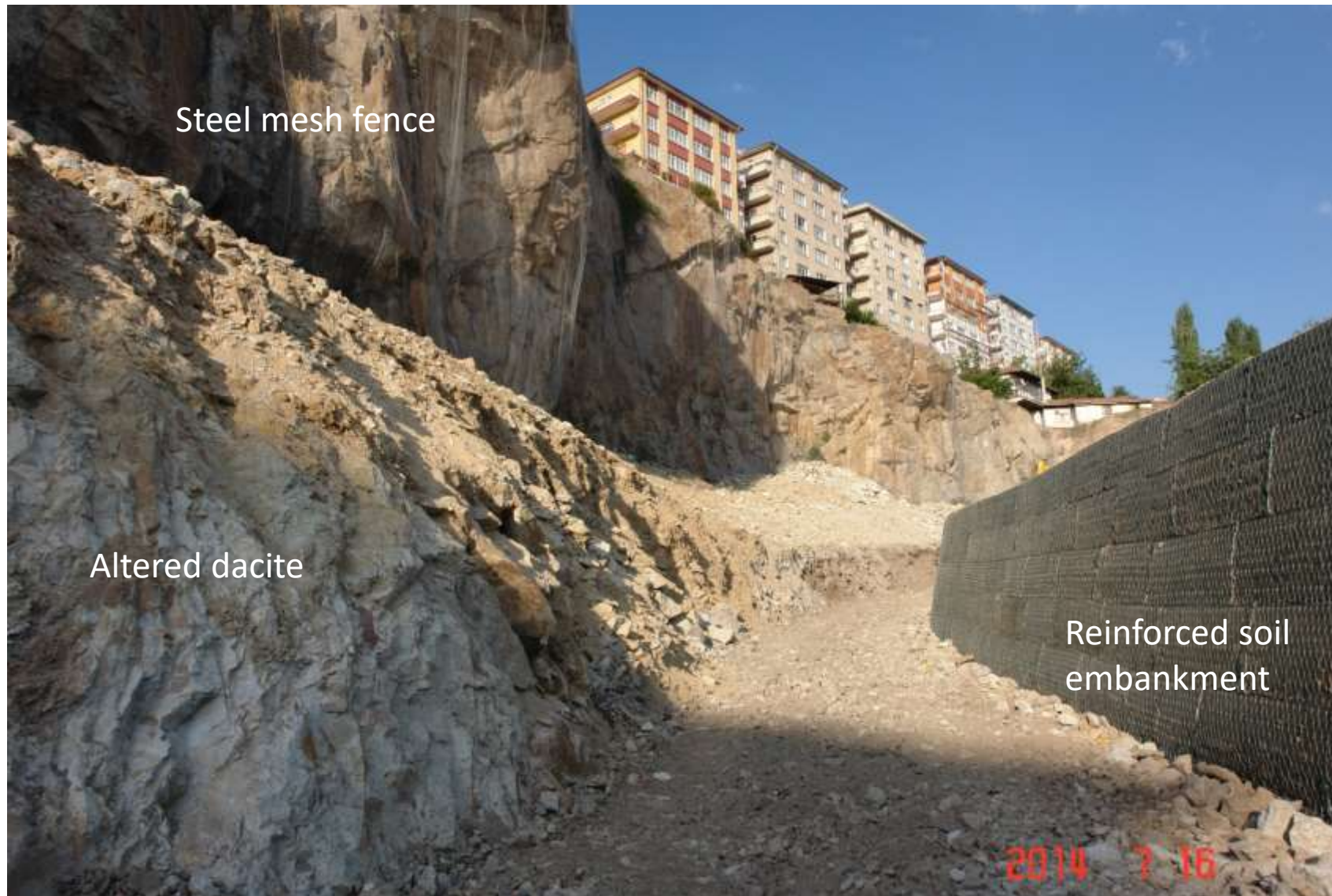
Remediation of rock material due to rockfall and instability with the use of compacted soil material. The project consists of rock material (dacite) , reddish soil and steel fence materials (Selçuklu District, Keçiören,Ankara. Photo courtesy of Kılıç, 2014)
