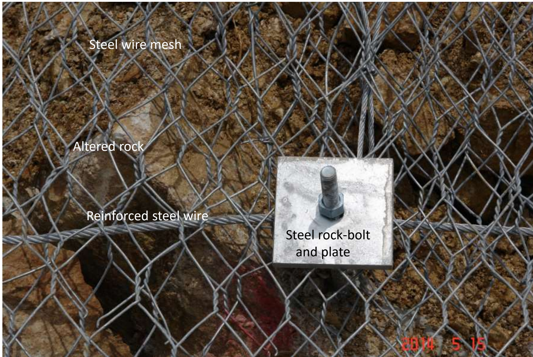
A closer view of the rock-bolt and wire mesh materials to prevent rock fall damage
