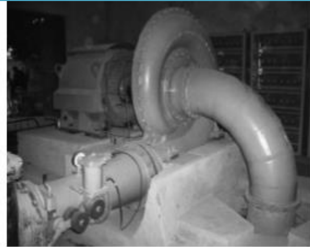
FIGURE 2.27 An induction generator coupled with a Francis turbine in a micro hydropower plant Afghanistan.
