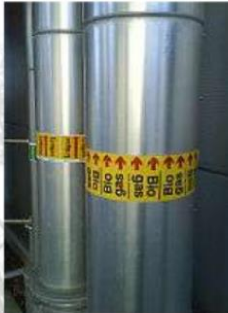
Pipes carrying Biogas
