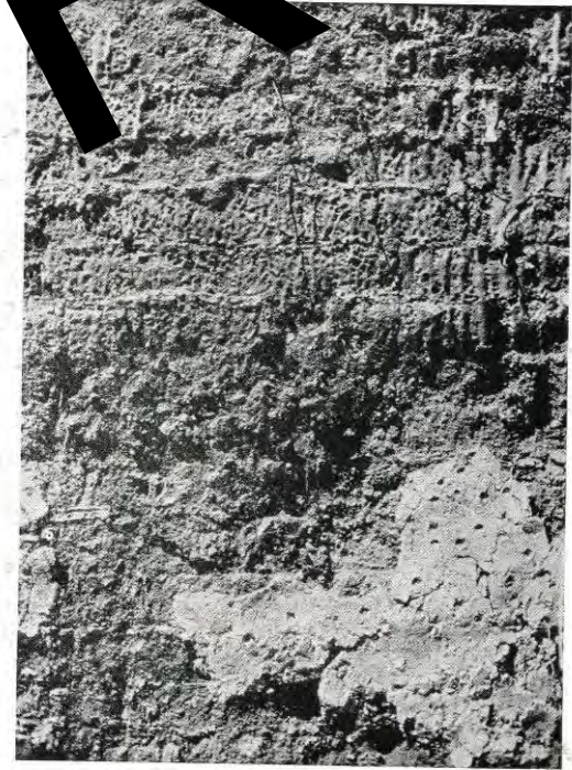
b. The staircase wall (room 3) showing vitrified brickwork: on the lower plaster is visible the finger-print keying for the intonaco
