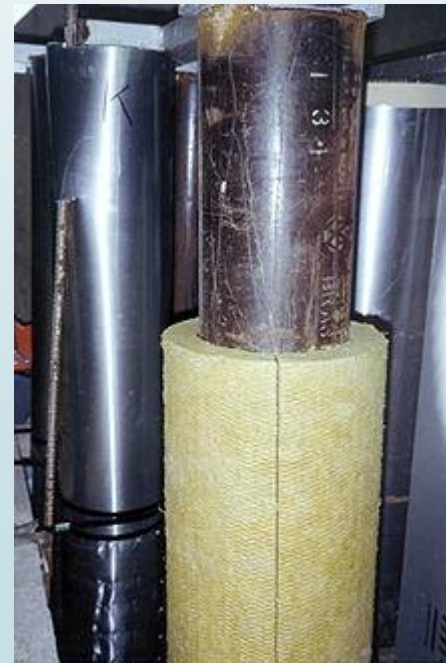
Pre-moulded rockwool pipe insulation in 1992 WH fire test. For small pipes, the insulation is in one piece and "snaps on". For larger pipes, the insulation is in two halves that are pressed together.
